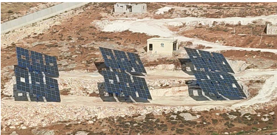
Figure 4. UNICEF-funded IYD Solar system in Harim
